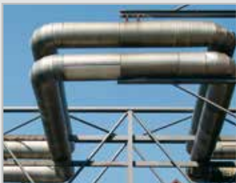
Pipelines subject to pressure
